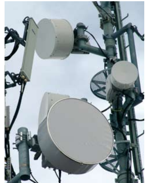
These directional antennae on the Jakobshorn (canton of Grisons) link mobile phone base stations and switching centres over relatively short distances.
