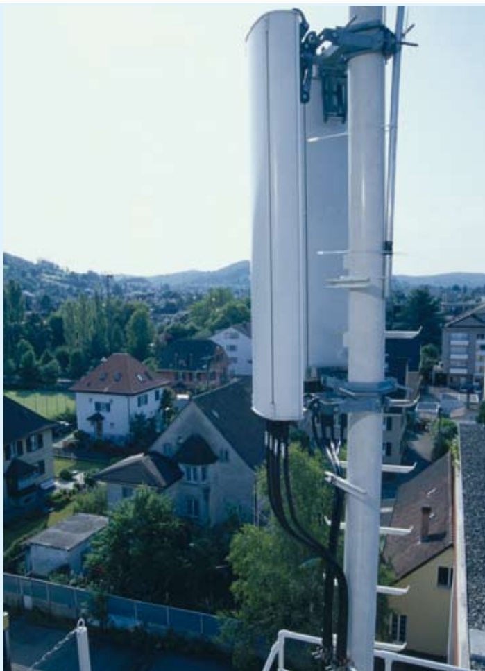
The antennae installed at base stations establish contact with mobile phones within their range.
