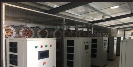
Installation full scale ~ 100 m 3 /h
