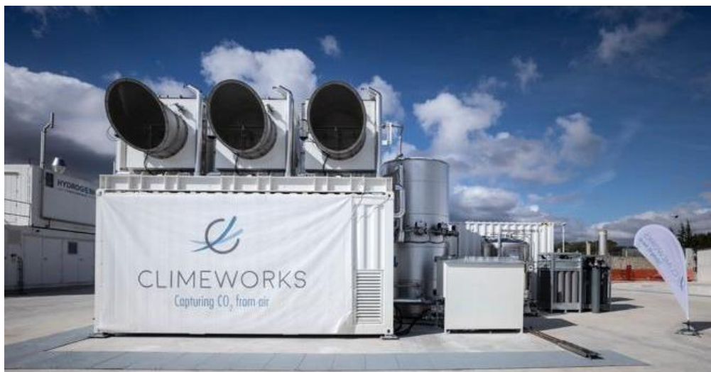
Figure 15. DAC 3 plant as part of STORE&GO. 81
