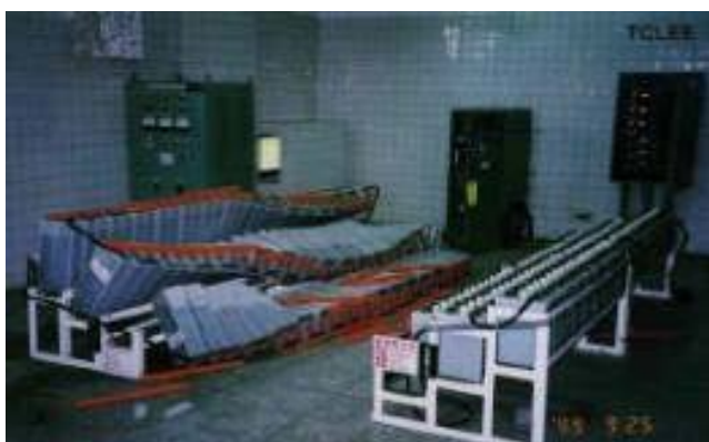
Schäden an Notstrombatterien (Chichi, 1999) 1
